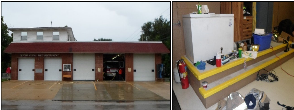
Fig. 4-12. Example of exterior (left) and interior (right) wet flood-proofing of a fire station.
